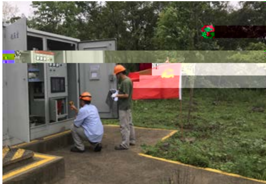
On the eve of the Super Typhoon Lekima's landing, the wind farms of Longyuan Jiangsu Company carried out special inspections to investigate and eliminate hidden troubles.
